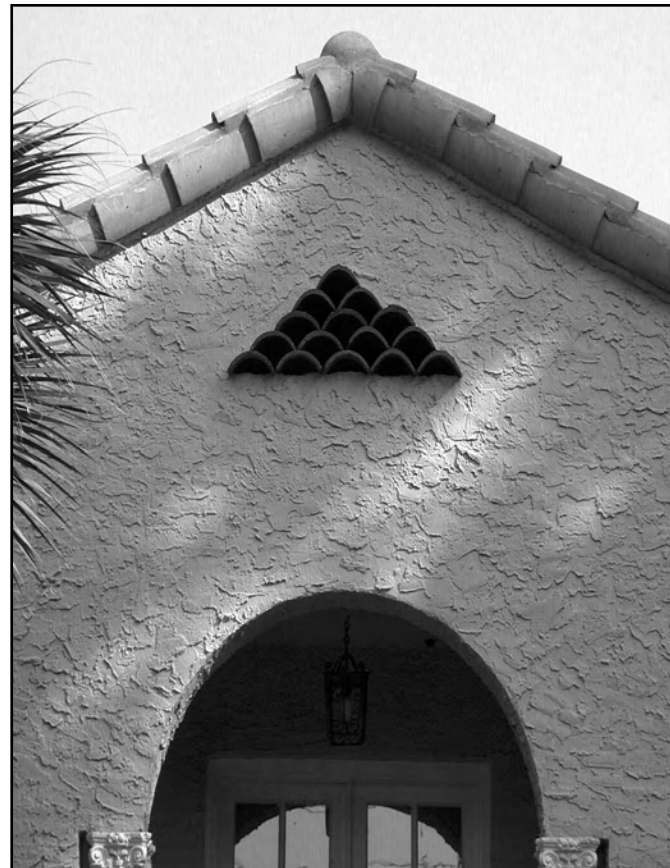
Gable end ventilation achieved with clay barrel tiles.
